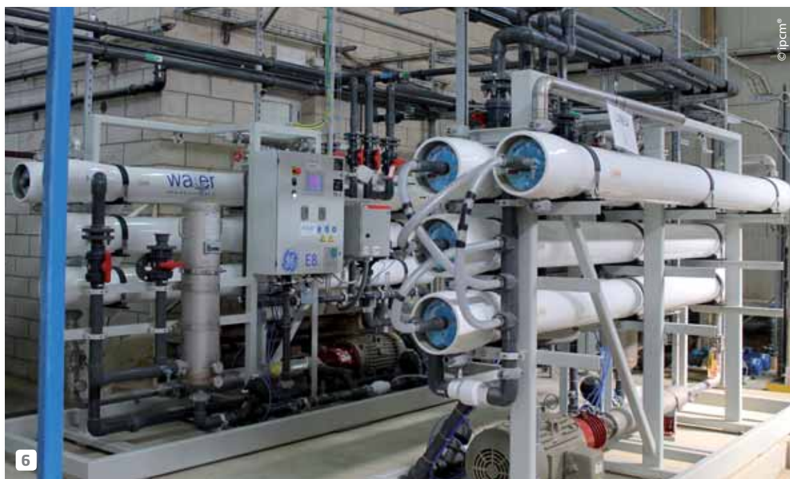
6 The two EDI lines. In the foreground, to the right, you can see the housings in which the membranes are inserted for the electro dialysis process.
