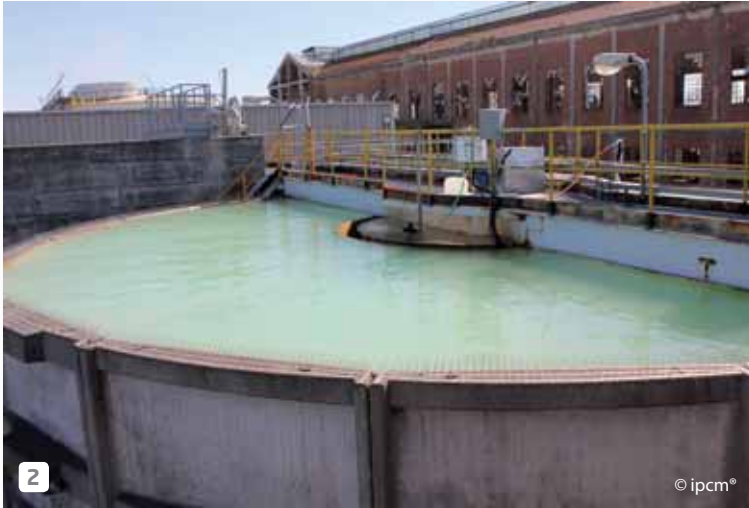
2 The sludge decanter of the physical-chemical treatment plant.
